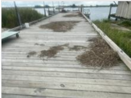
Figure 2. Flooding of the former HSRL dock on a spring tide during October 15, 2014 prior to elevating it in 2007 (upper image). Debris deposited on the dock from storm surge following Hurricane Isaias in August 2020.
